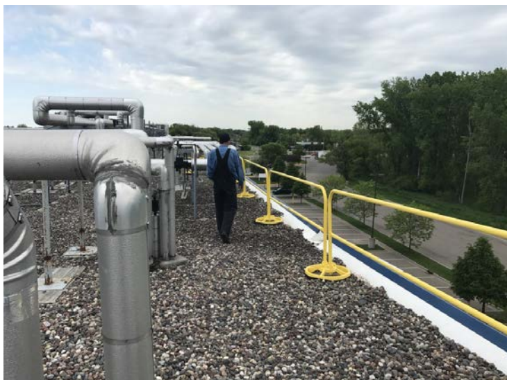
Passive System - Guardrails
